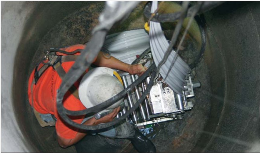
A spiral-winding machine located in an existing manhole creates a new Expanda pipe.
